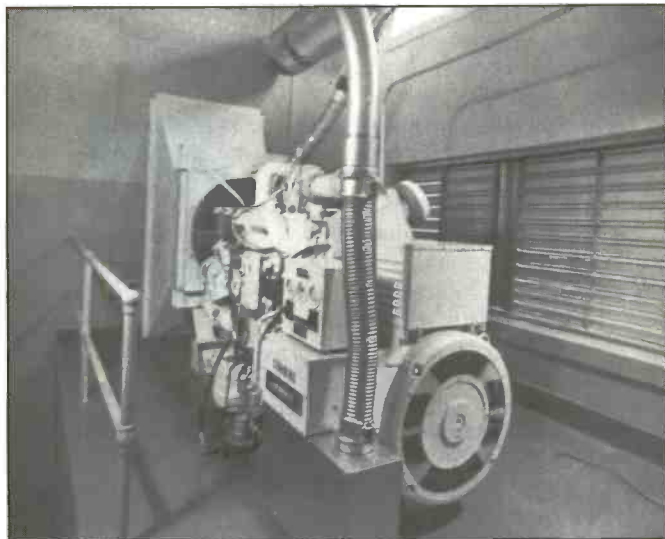
Here's a photo of an old 1960s Cold War-era generator shortly after its installation. (All photos by Larry Cornelison)
