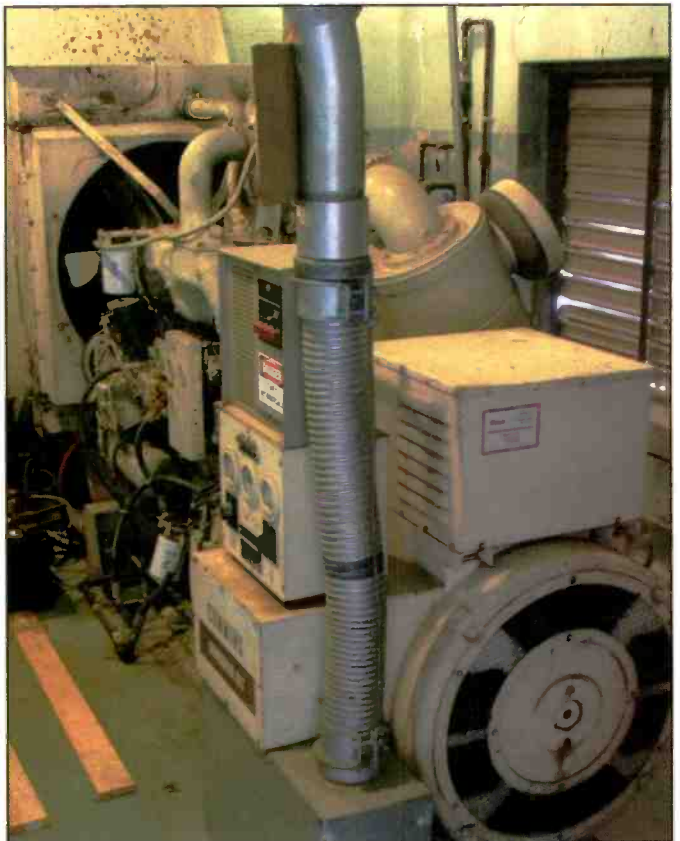
Another photo of the generator—it still works!
